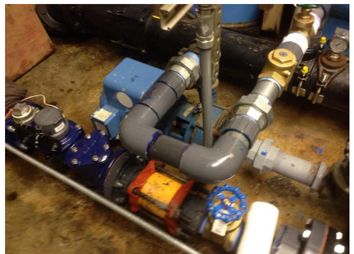
SECONDARY DISTRIBUTION AFTER CONVERSION PRIMARY AND SECONDARY PUMPS CAN NOW OPERATE INDEPENDENTLY
