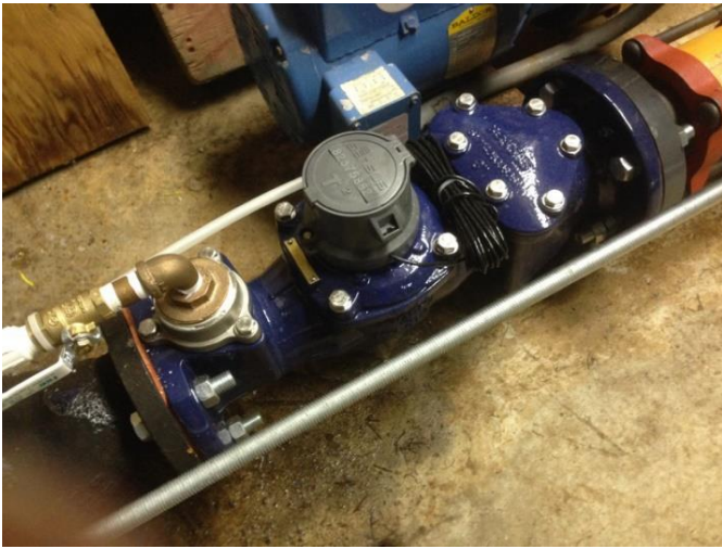
THE NEW METERING MEASURES ALL WATER FLOW INTO THE DISTRIBUTION SYSTEM AND SENDS SIGNALS TO MISSION COMMUNICATIONS FOR ONLINE DISPLAY
