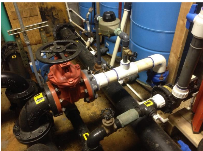
SECONDARY DISTRIBUTION PLUMBING BEFORE CONVERSION
