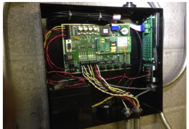
MISSION COMMUNICATIONS AFTER ADDING ELECTRONICS FOR METER
