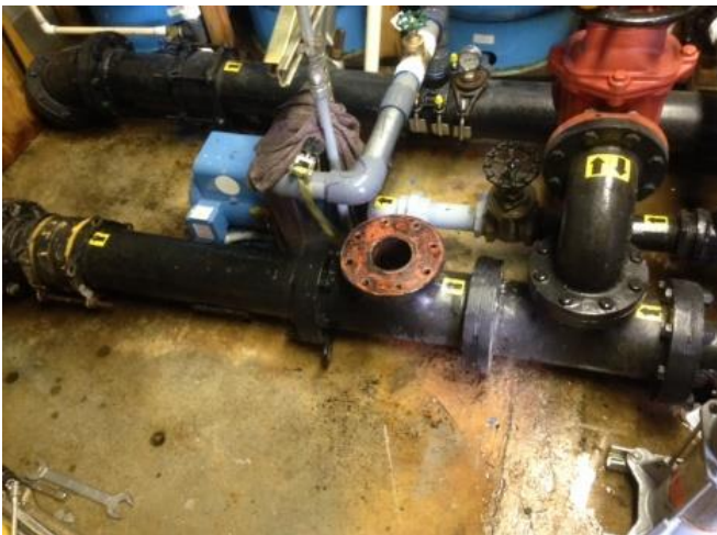
THE FORGROUND LEFT IS THE 6" DUCTILE IRON PIPES BEFORE CONVERSION - NEW METER GOES HERE
